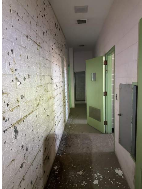
Architecture/Structural – Typ. Interior Block Moisture Blow-outs
