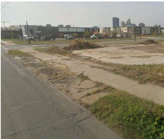
Figure 14 Broken sidewalk along the Front Street
