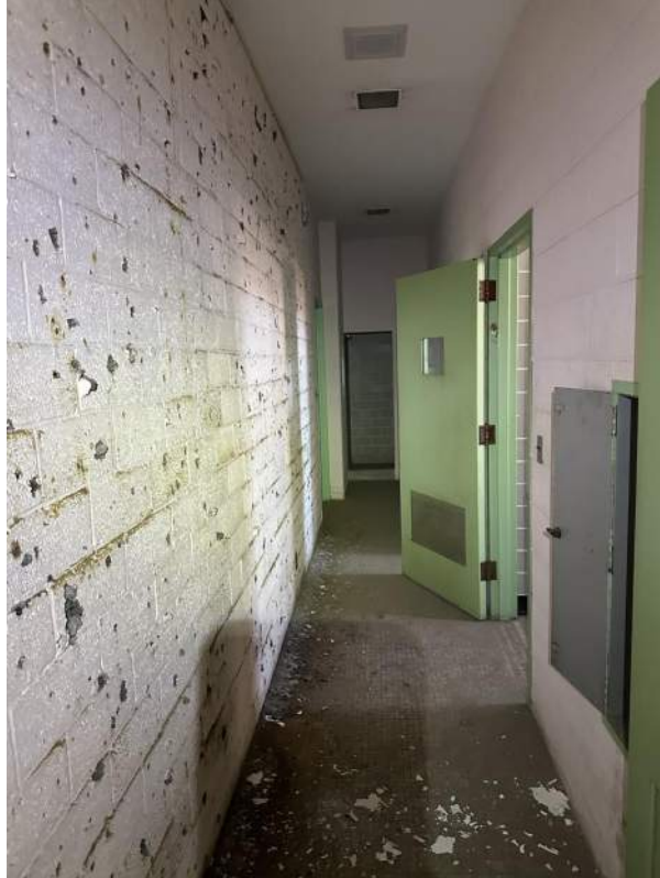
Architecture/Structural – Typ. Interior Block Moisture Blow-outs
