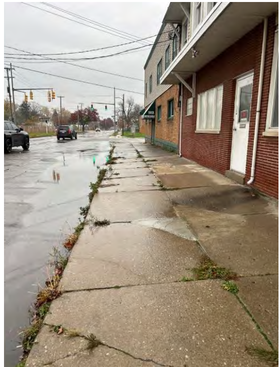
Figure 9 Clogged Road and uneven sidewalk
