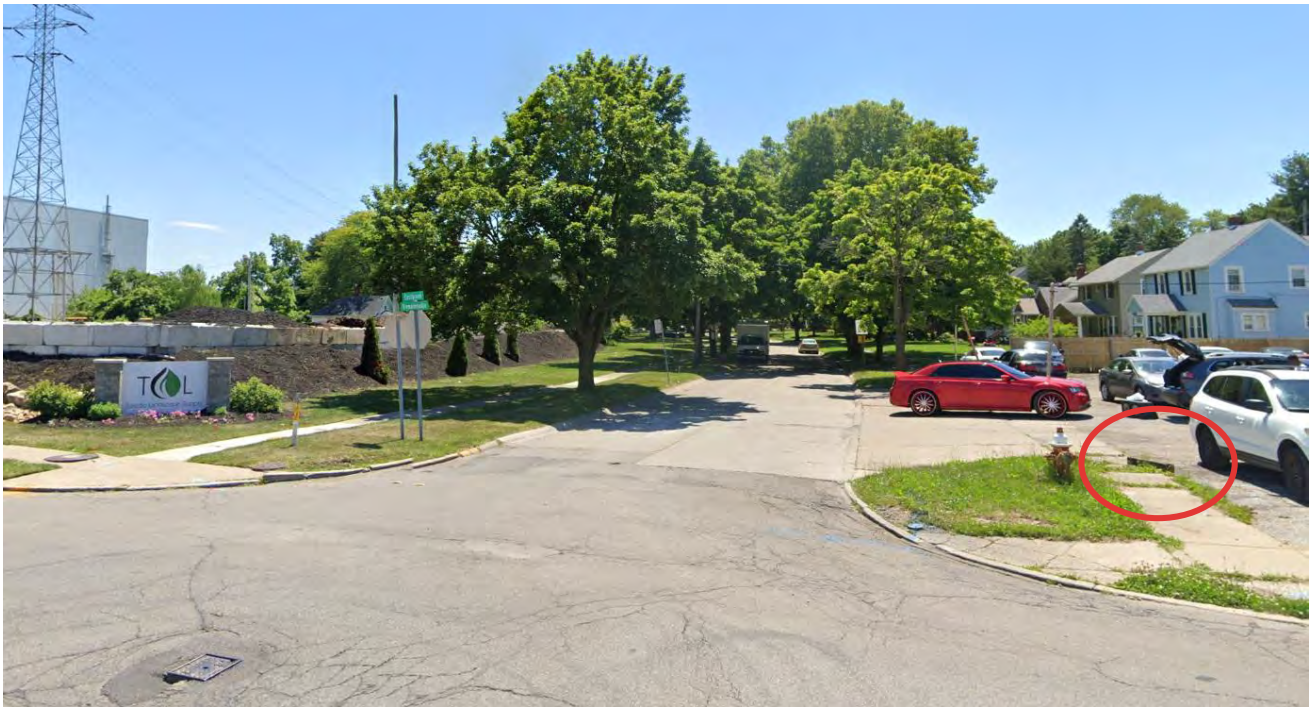
Figure 8 Missing ADA accessible ramps and raised manhole in middle of the sidewalk
