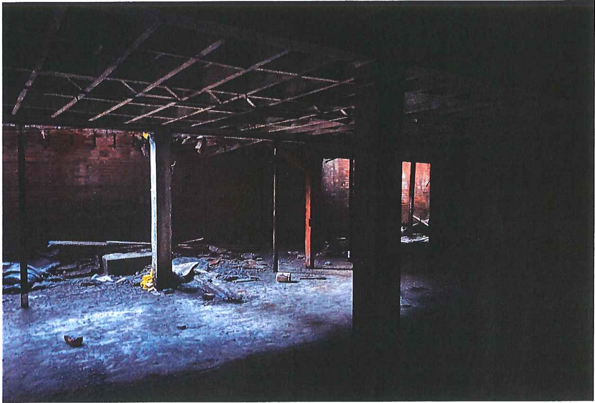
Plate 15: Basement, looking west-northwest towards collapsed ceiling.
