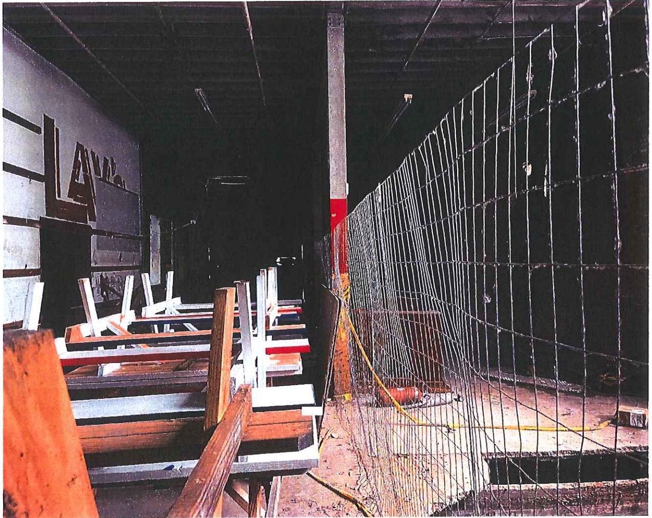
Plate 9: First floor garage/storage space, looking southeast towards garage entrance with collapsed floor to the right.
