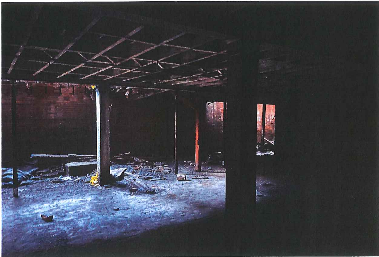
Plate 15: Basement, looking west-northwest towards collapsed ceiling.
